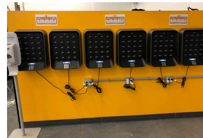
MakuSafe charging station.
