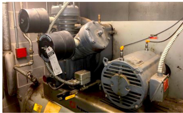
Figure 11: Motor vibration sensors installed on Ivy Tech’s second floor air compressor.
